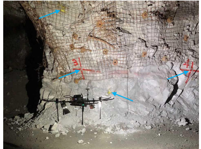
Fig. 4. Control points marked on the rib of the mine drift marked with spray paint (in red) and marked using a paintball gun (in yellow).
