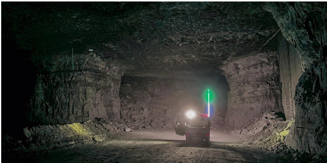
Figure 43 Boundary of mine cave-in from 2021 collapse of multiple pillars
